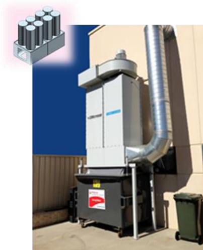
VC8 with dump bin Outside location
